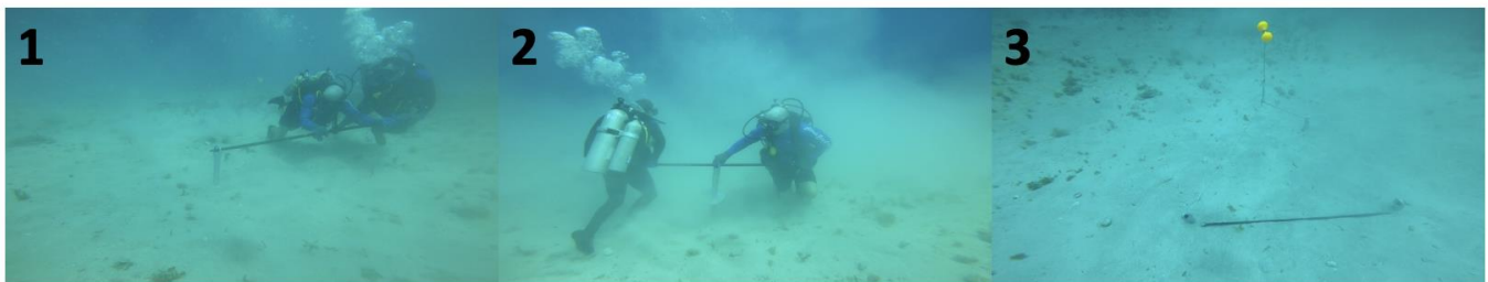
Figure S20: Three sand anchors are installed in a triangular arrangement to provide redundancy in holding power. To install the anchors, the lower disk of the sand anchor is first buried in the sand, and then a long turning bar placed through the anchor eye is used to twist the anchor into the substrate until only the eye remains above the sand.
